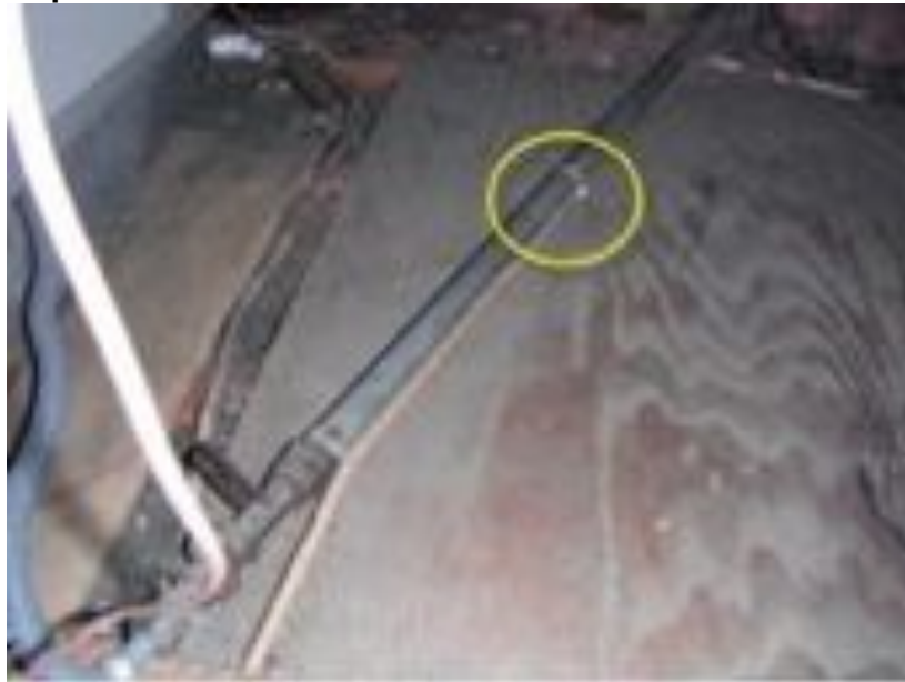
ROMEX cables must be protected from the metal cabinet with a grommet; abrasion can lead to the insulation being cut
