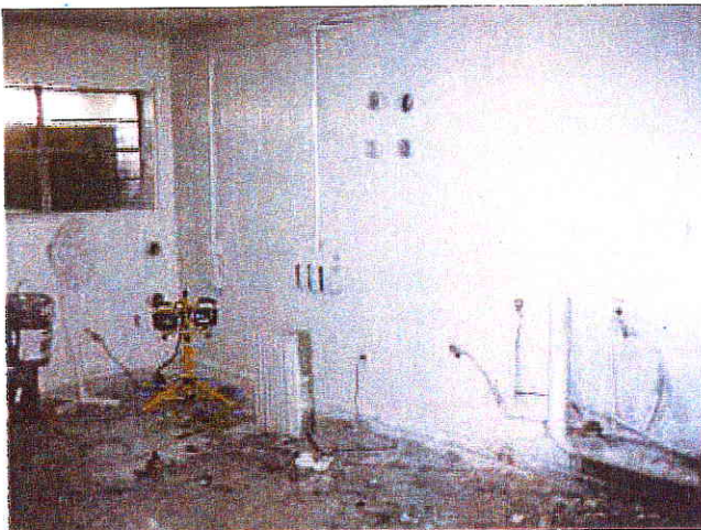
Common Laundry (Fire Damage)
