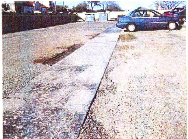
Parking Area Deferred Maintenance
